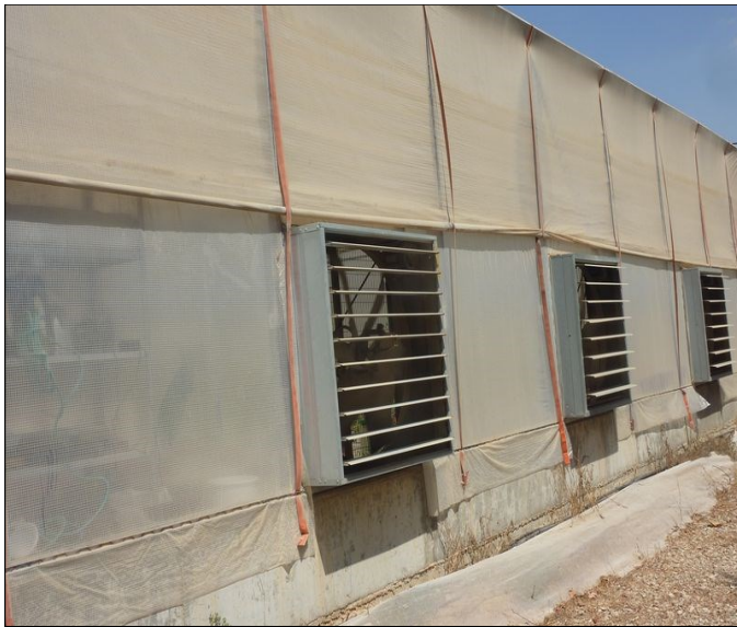
Fig. 18. Greenhouse ventilation system.
