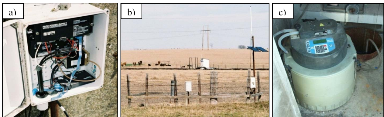
Figure 2. Selected hydrologic instrumentation at the Riesel Watersheds; a) Campbell Scientific data logger and telemetry radio and modem, b) rain gauge station with a tipping bucket and standard gauge and radio telemetry equipment, and c) ISCO autosampler.
