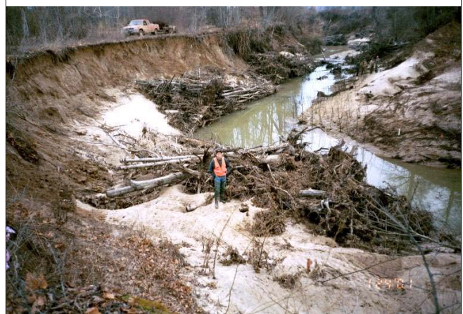
Figure 1. Typical meander bend along Little Topashaw Creek, Mississippi shown just prior to, during, and six months after placement of large wood structures.
