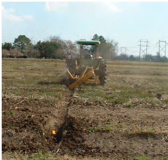
Figure 1. Installation of semi-circular quarter-drain, perpendicular to sugarcane furrows, using a PTO-driven circular cutting trencher blade to remove soil.
