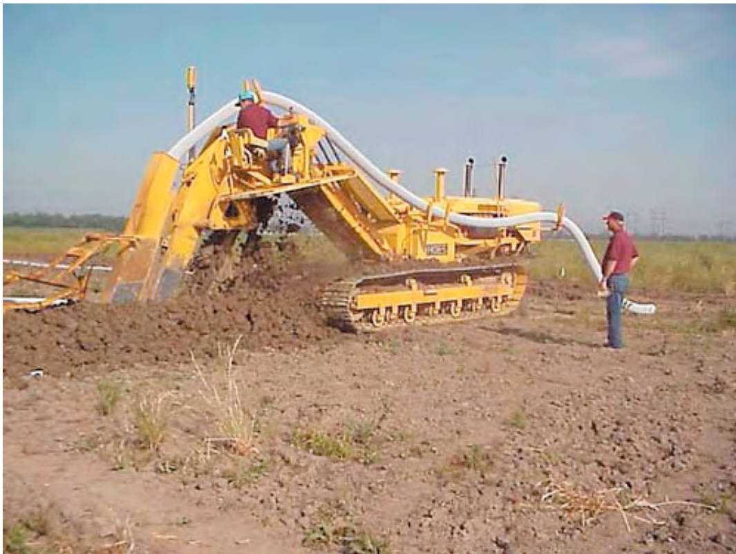
Installation of subsurface drainage system at St. Gabriel, LA using a chain-type trencher with laser grade control.
