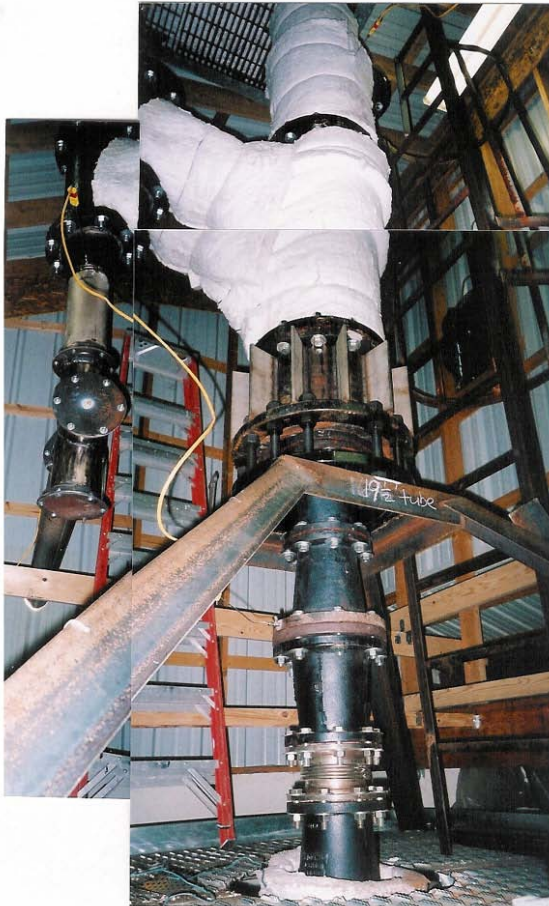
Pilot gasification reactor Western Research Institute Laramie, WY
