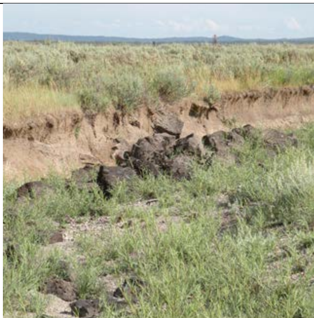
Figure 33. Historical Rip-rapping, Dry Creek, Henninger Ranch
