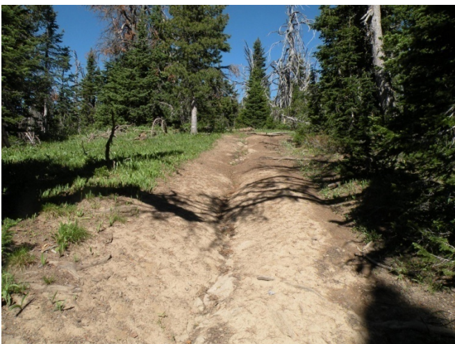
Figure 10. Road Ruts on Road to Blair Lake
