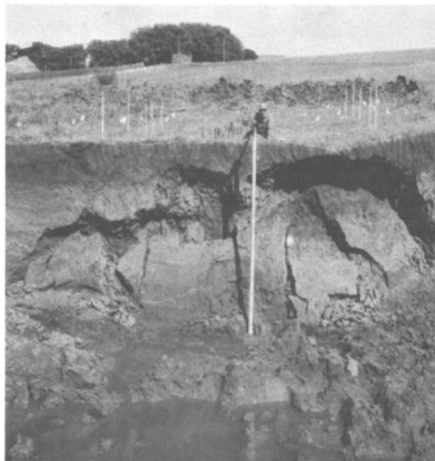
Fig. 1—Large alcove failure along gully bank.
