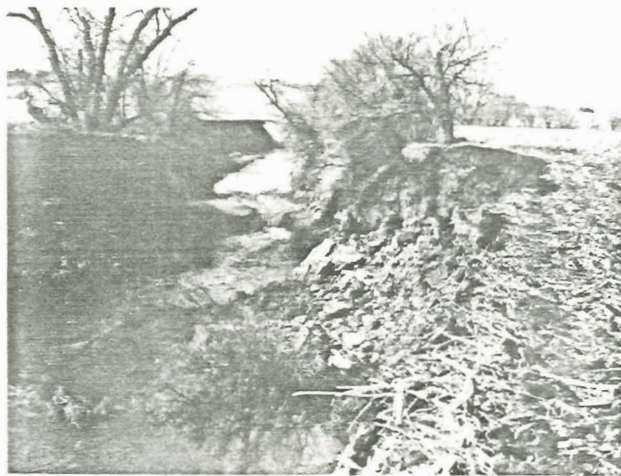
Figure 2.--Active erosion scarp causing channel degradation and enlargement, Keg Creek, Iowa
