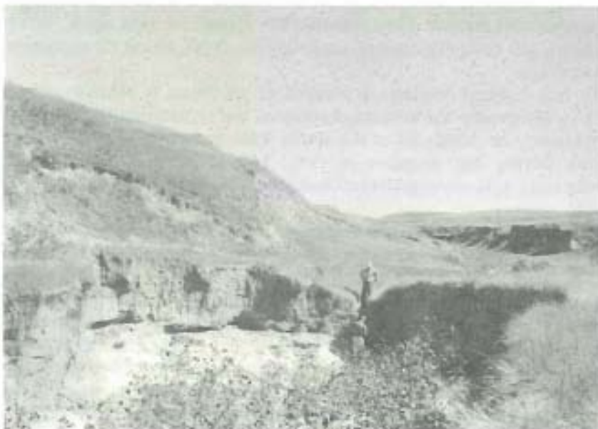
Figure 31.--This photograph, taken September 2, 1960, shows the overfall at item 3A (3,500 feet downstream from item 3). Downstream the channel has entrenched an additional 12 to 15 feet. Upstream the bottom has become stable and is covered with grass. The bank remnant from the channel erosion cycle now active in item 3 (above photo) is shown on the right, upstream.
